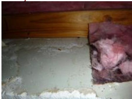
13 - water damage (dry)
