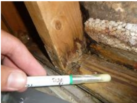
13 - mold like growth and surface sample
